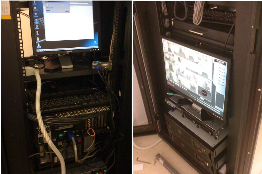
Image 3: Workstation server for IBSS (left); CCTV monitoring server (right)
