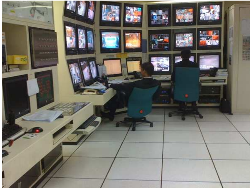
Image 7: Control room for IBSS (KLCC)
