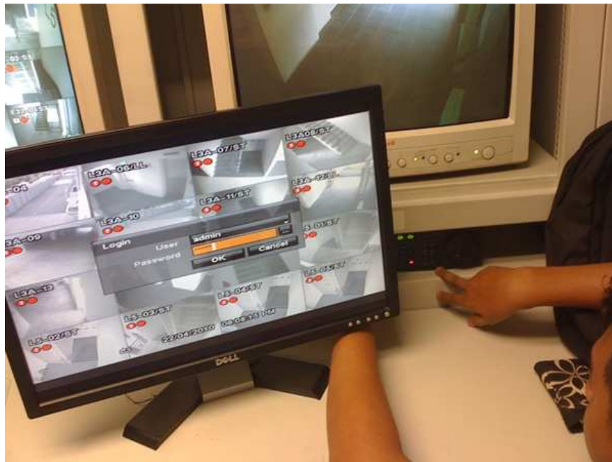
Image 8: Doing troubleshooting on malfunction monitor
